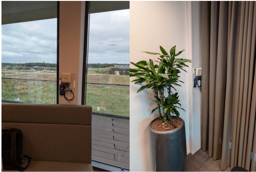
Figure 21. Photos of the Channel Sounding access points installed at the Vitality Hub.
