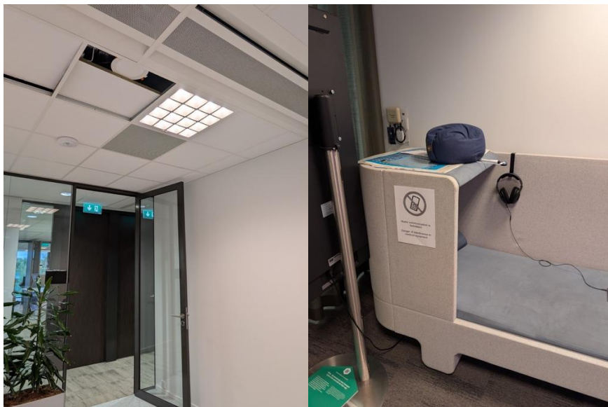
Figure 20. Access Points installed at Vitality Hub.
